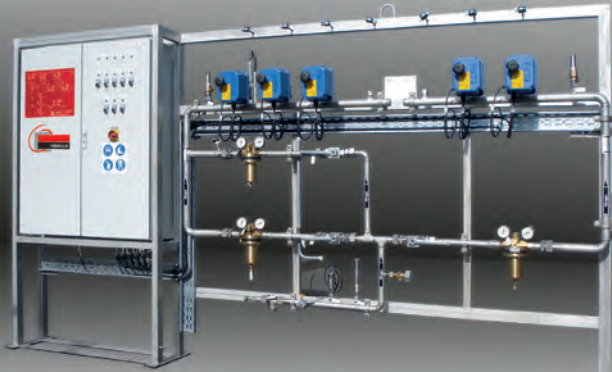
N 2 Valve station
