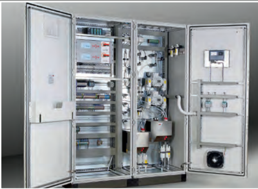
Gas analyser cabinet
