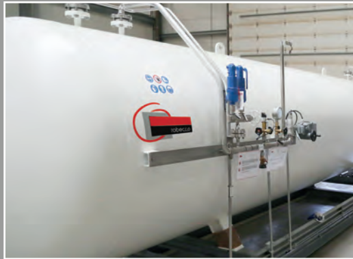
CO 2 high-pressure tank
