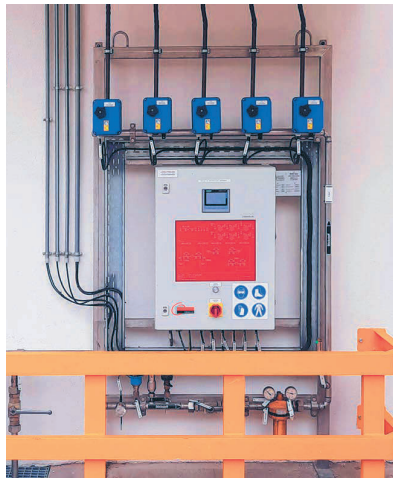
Figure 3: N 2 valve station for sewage sludge silos
