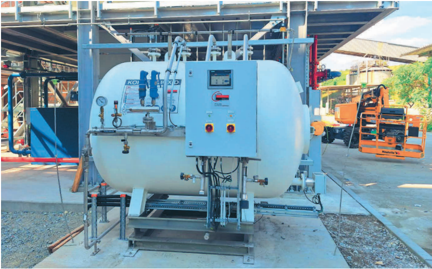
Figure 1: CO 2 storage tank
