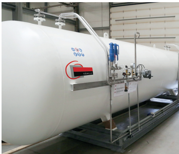
Figure 2. CO 2 high-pressure tank.
