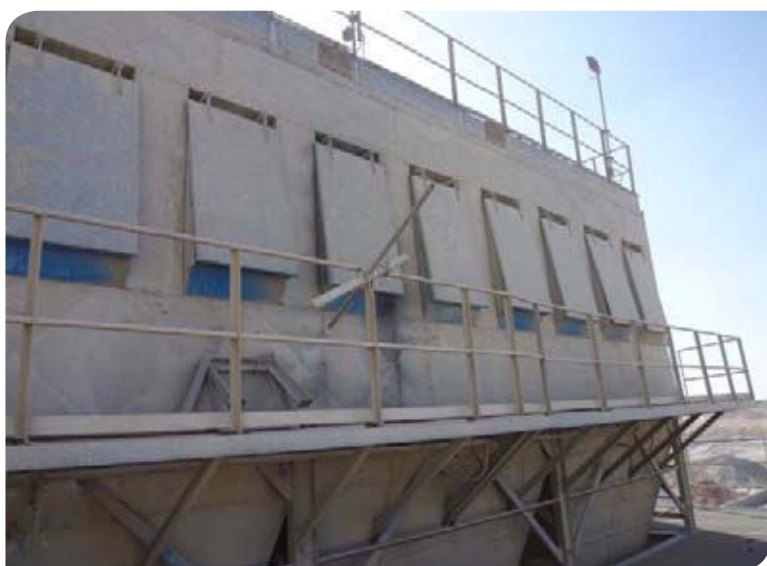
Below: Non-type tested explosion venting devices mounted on a bag house of a coal grinding plant. This does not conform to required norms and will lead to heavy bag house damage in the event of an explosion.
