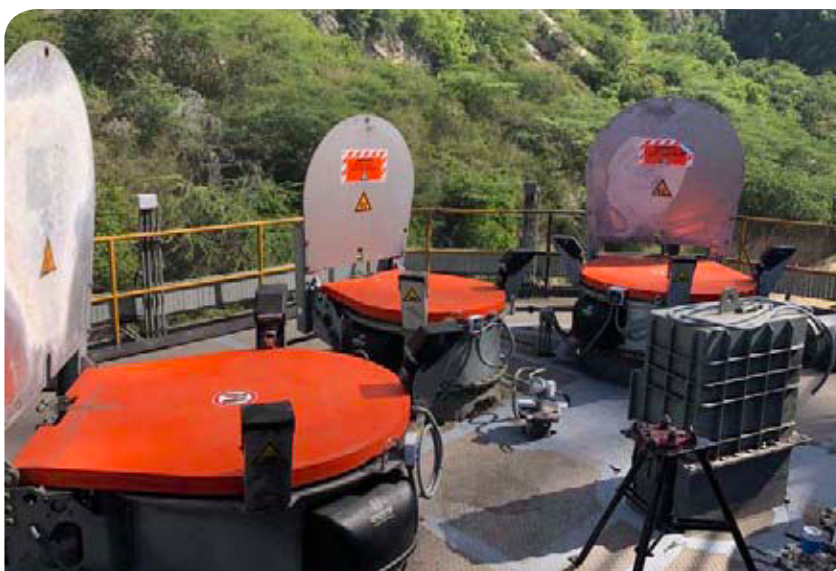
Below: Thorwesten Vent's self-reclosing explosion vents on top of a pulverised coal silo.
