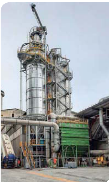
Below: robecco inerting system (left) and control cabinet (right), recently installed for a client in the global cement sector.
